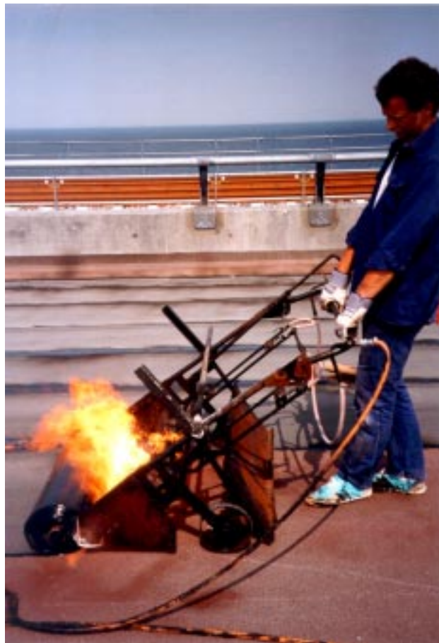
Figure 2. Polymer modified waterproofing sheets are torch welded to the surface of the primed concrete.
