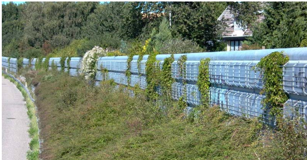
Figure 3.32. Steel noise barrier with steel grid to support vegetation on the barrier at Highway M14 north of Copenhagen, Denmark.
