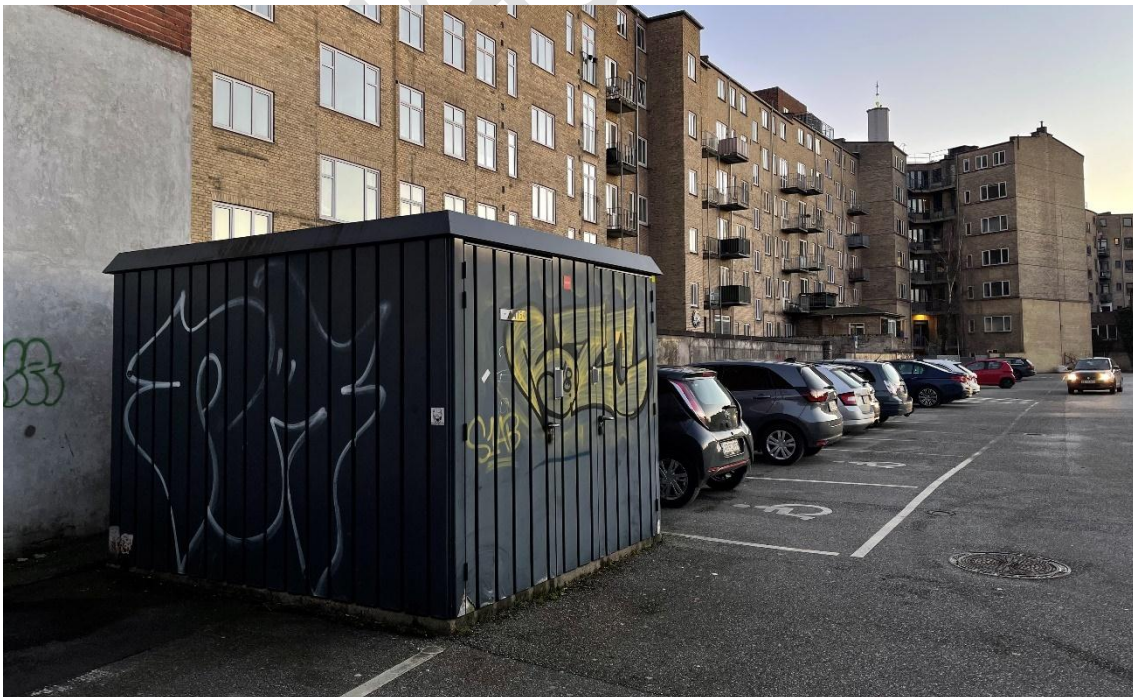
Figur 6.7 Transformerstation i Aalborg. Foto: Rambøll.
