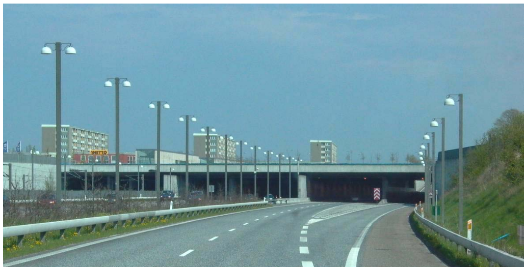
Figure 4.5. 700 m long section of the new highway to Copenhagen airport, Denmark was constructed as a cut and cover strategy in order to reduce the noise exposure for some nearby multi-storey apartment buildings.
