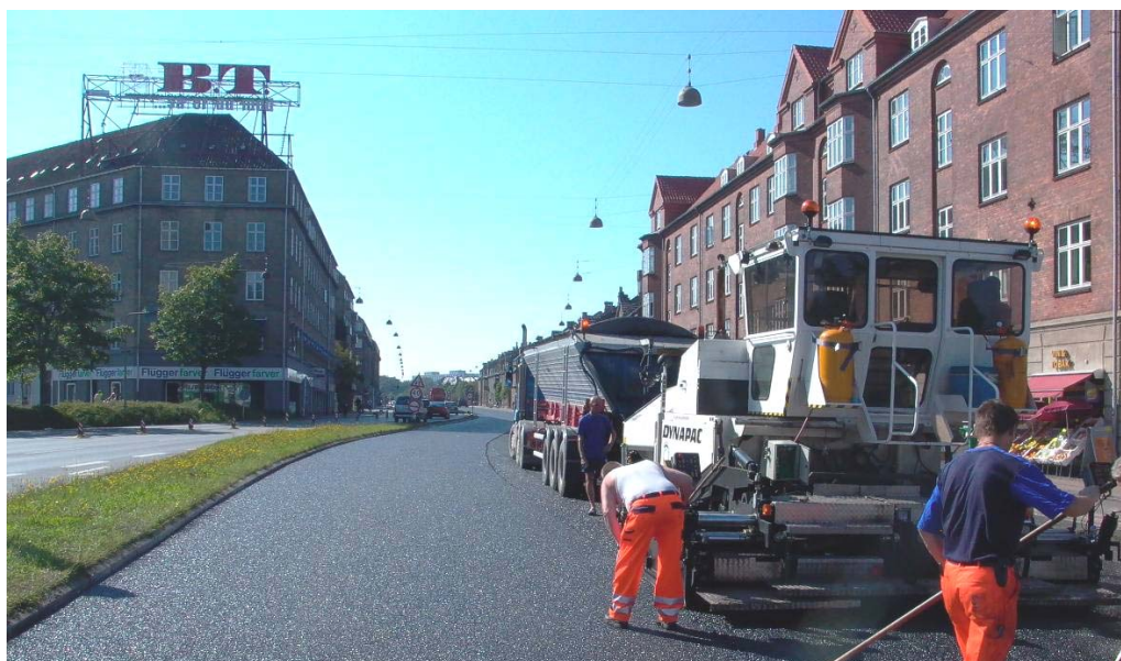
Figure 6.6. When the pavement on an existing highway has to be replaced, the road administration might consider using a new noise reducing pavement type. Here noise reducing two-layer porous asphalt is applied on a highway in a densely built up area in the municipality of Copenhagen.
